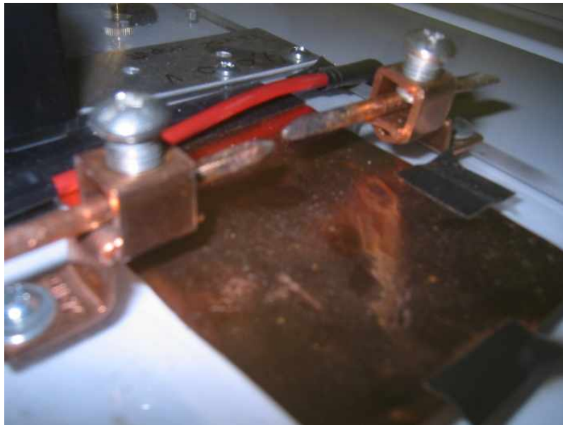
Spark Gap using 2 large copper wires and Electrical box fasteners
